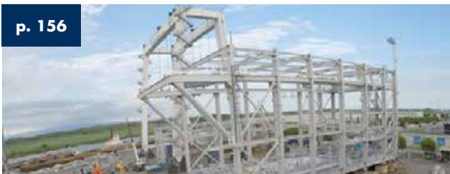
On Shore modules Upper Zakum Oilfield - UAE - 6 modules
