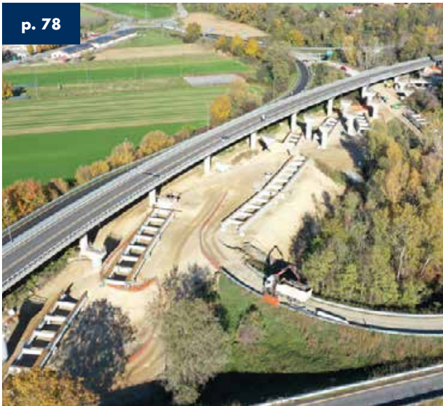
Fossano Bypass Viaducts Road S.S.231 "di Santa Vittoria"- Italy - 780 m total length
